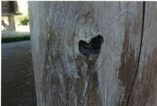
③ 節の腐朽落脱
