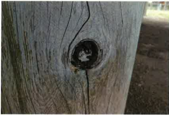
① 節の腐朽落脱
