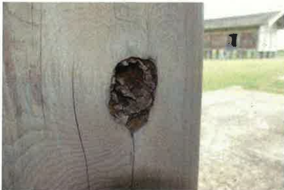
③ 節の腐朽落脱
