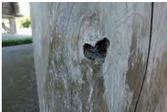
③ 節の腐朽落脱
