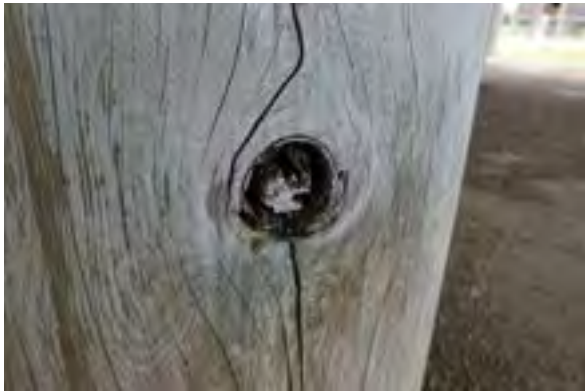
① 節の腐朽落脱
