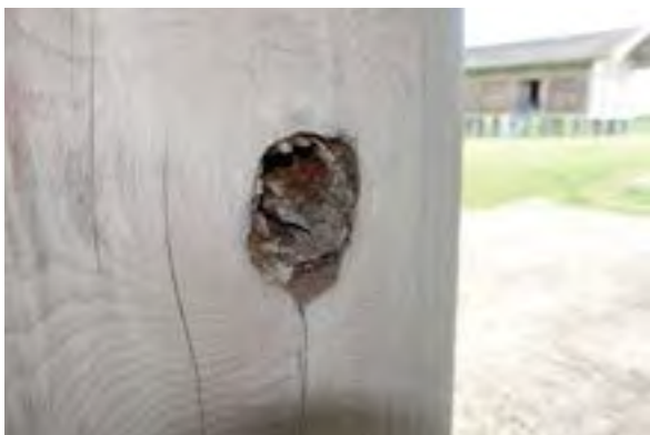
③ 節の腐朽落脱
